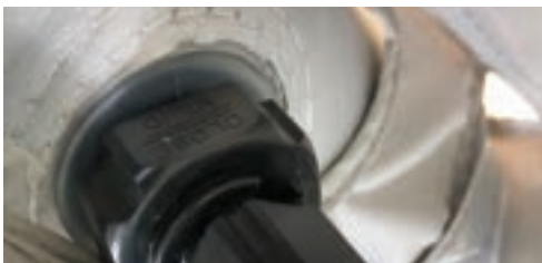
To OPEN valve turn counter clockwise. To CLOSE valve turn clockwise until firm.
